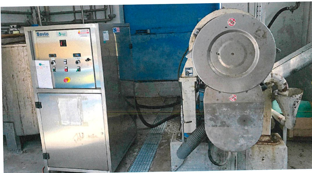
◀ The AST installed at Sofidel, Via di Leccio.
